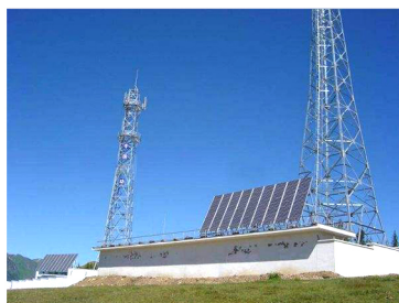
communication base station
