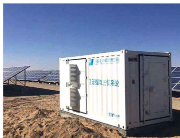
Photovoltaic energy storage system
