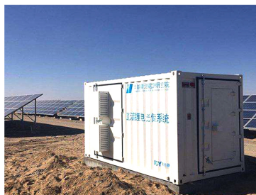
Photovoltaic energy storage system
