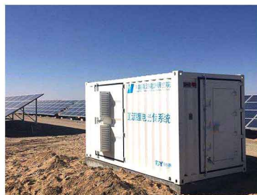
Photovoltaic energy storage system
