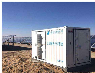
Photovoltaic energy storage system
