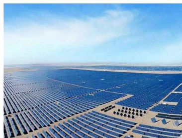
Photovoltaic power station
