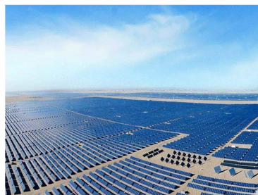
Photovoltaic power station
