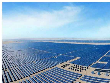
Photovoltaic power station
